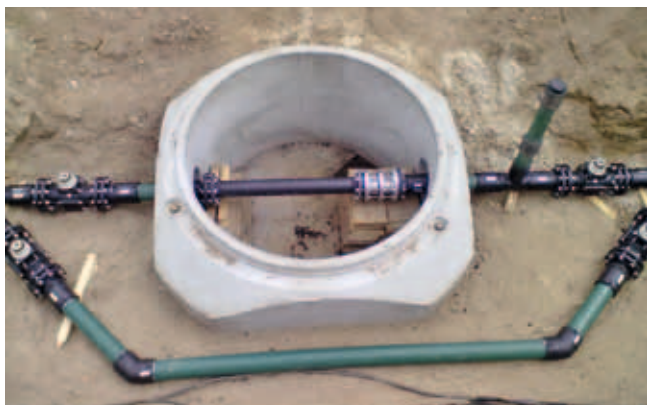
Figure 1: Testing point to monitor incrustations in the vacuum system. Photo: HAMBURG WASSER
