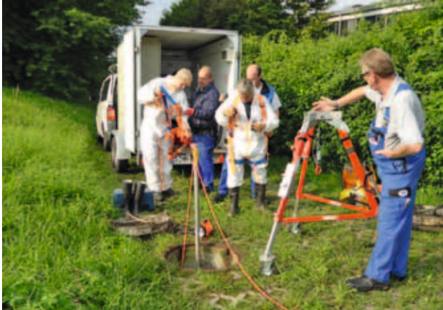
Figure 2: Installation of a measuring station for quality testing at a stormwater overflow basin. Photo: Stuttgart University, ISWA
