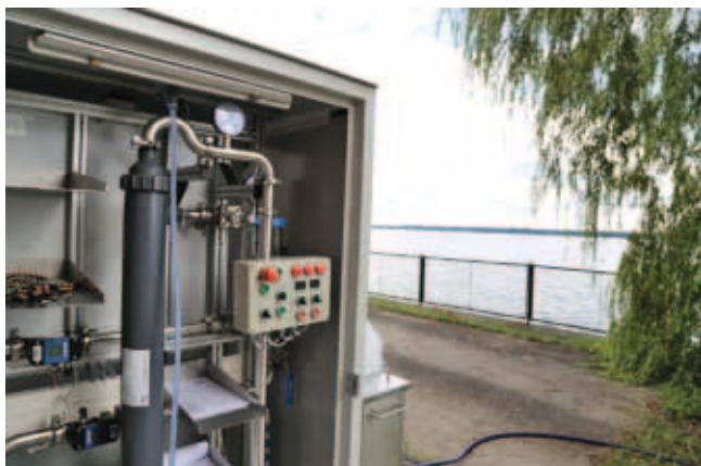
Figure 2: Model plant for continuous cross-flow ultrafiltration at the waterworks in Friedrichshagen, Berlin. Photo: Daniel Karthe
